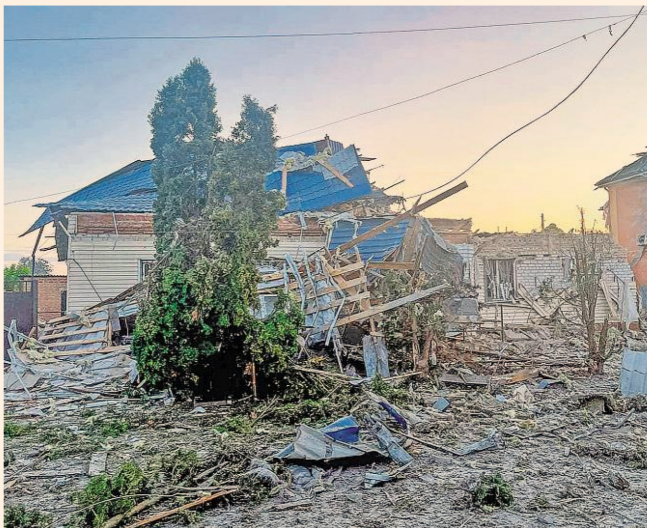
Wrecked: a house in the city of Sudzha, Kursk, said to have been shelled by Ukrainian forces — Kursk governor/Telegram/AP
